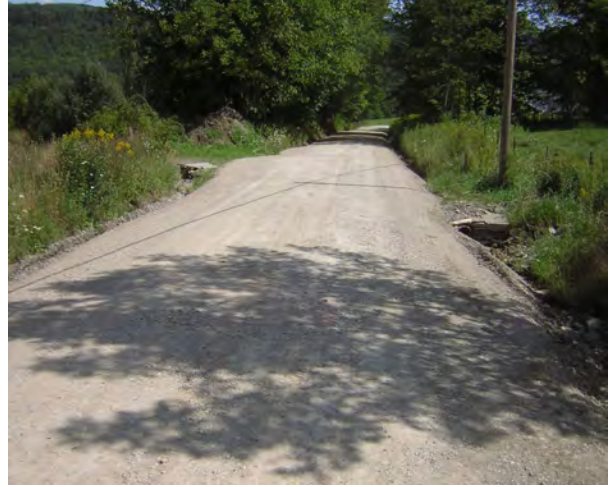
A new cross pipe on Mattes Road in Choconut Township helps to reduce erosion by breaking up the volume and velocity of runoff
