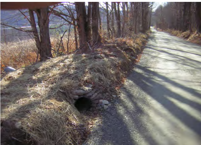
A through-the-Bank pipe on Hall Rd in Forest Lake Township takes water off the road in order to reduce erosion
